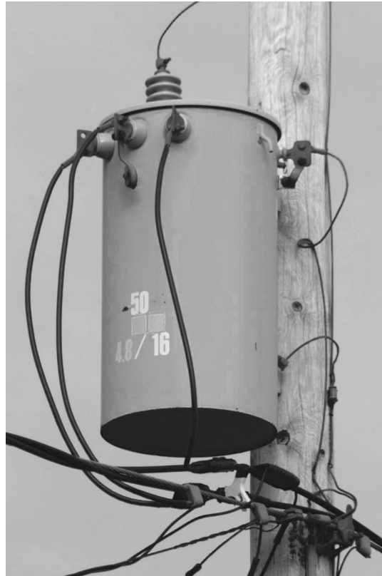
Figure 1. Power transformers are often used in power distribution lines.
