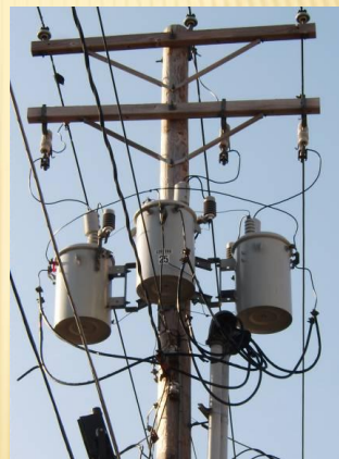
Three Phase Bank Three individual Transformers
